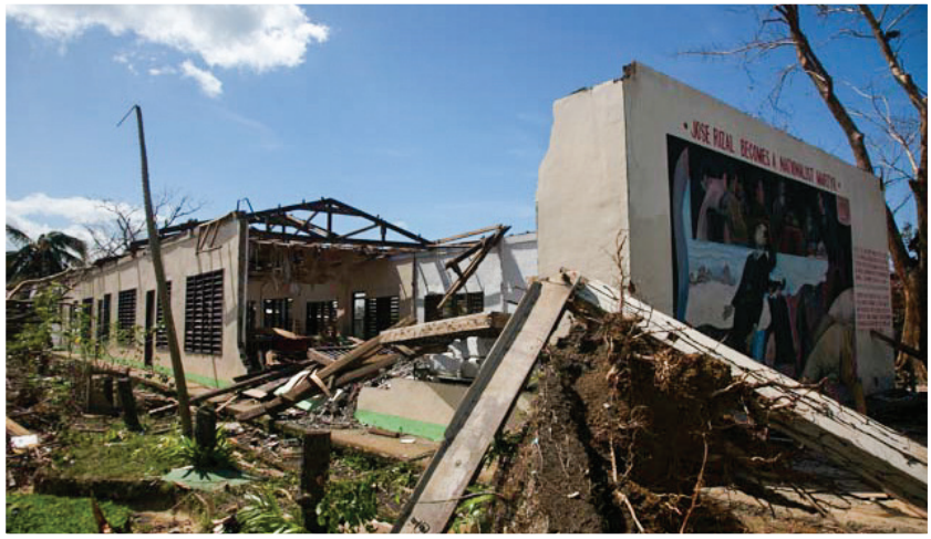
UFI's four new classrooms at President Roxas East Elementary School, completed in Nov 2014 with comparison of the old destroyed building following Typhoon Yolanda a year earlier.
